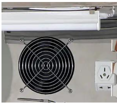
Lighting system and BOD socket
